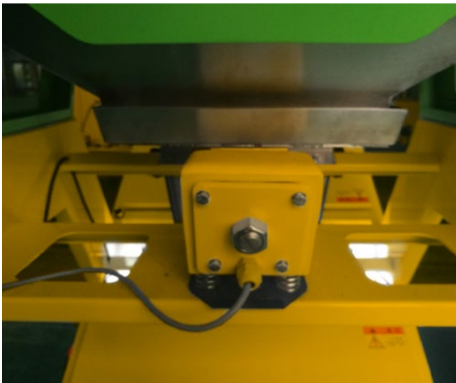
Dust and foreign matter of vibrator platform and vibrating bucket
